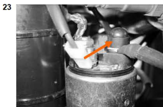
Step 23: Cover required on starter motor and alternator connection nut (positive feed).
